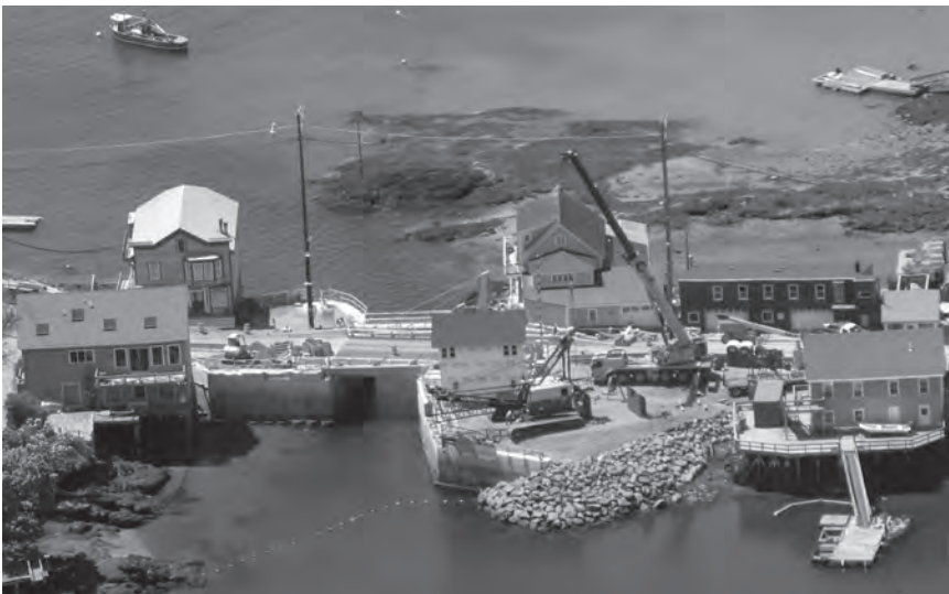
Above: Coast Guard photo taken after removal of temporary bridge. Upper right: New bridge span is raised for marine traffic, 5/27/16 Lower right: First boat goes through the passage, 5/27/16
